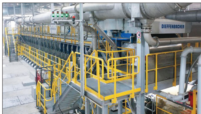
A Dieffenbacher CPS+ continuous press in a particleboard plant.
