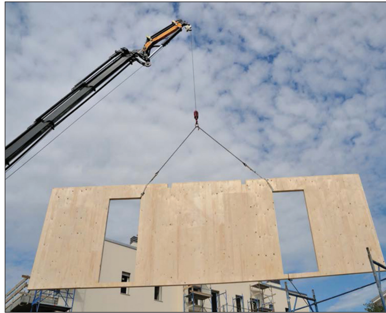
The great timber construction boom is also due to the possibilities of automation and a higher degree of prefabrication.
