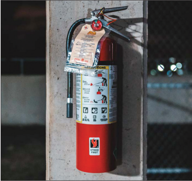
Fire extinguishers are considered part of the active fire protection system (Image: Erik Mclean/Unsplash)
