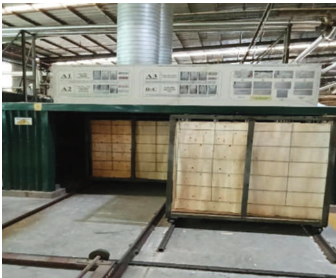
Vertical stack dryers.
