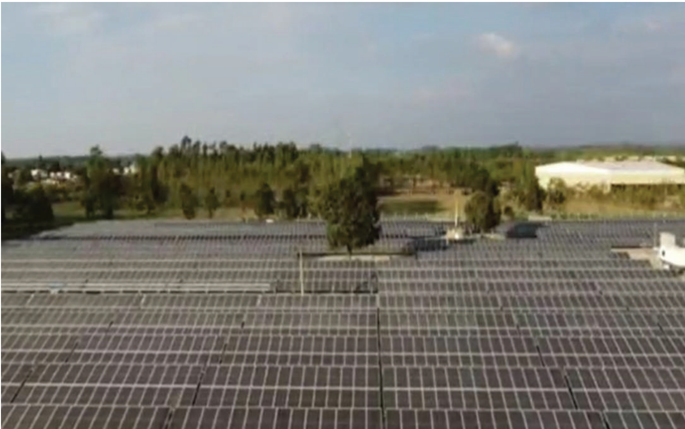
Rooftop solar installation at Century Plyboards manufacturing facility — driving renewable energy targets.
